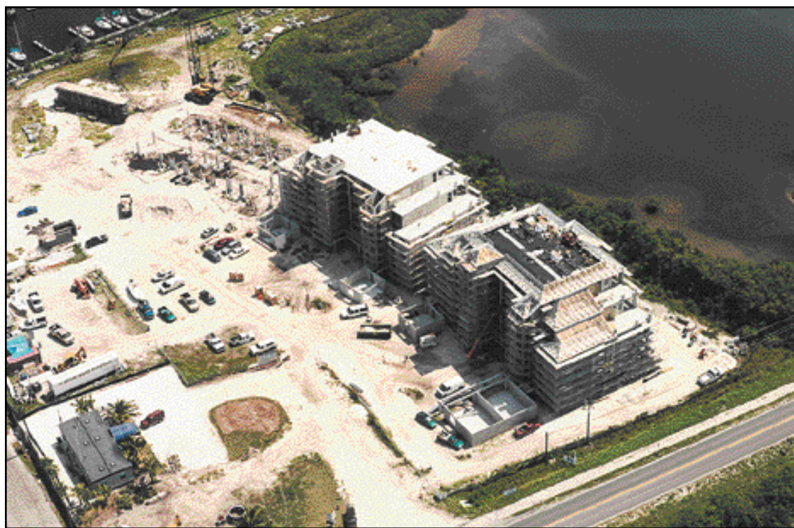
The Boca Vista Condominiums in Boca Grande, currently under construction, are situated on the waterfront of Charlotte Harbor. The five buildings boast 20 units each. Kellogg & Kimsey of Sarasota is serving as the construction manager and general contractor for the project.
